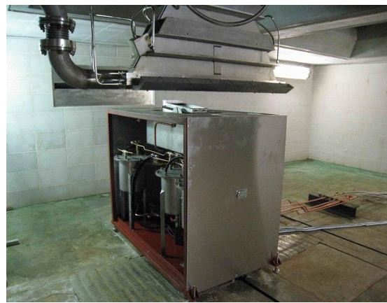
Fig. 2 Reactor for irradiation of transformer oil.
